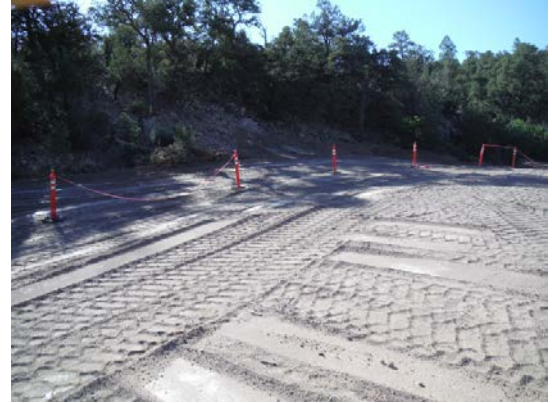
The area was kept cordoned off pending soil analysis results.
