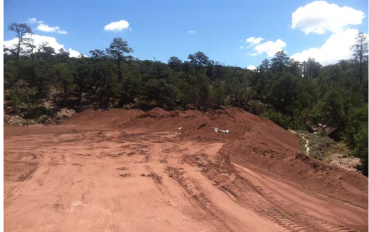
This Photo shows the area on the eastern boundary of the SSL area where stockpiles SKPL-0088 and SKPL-0089 were dumped.
