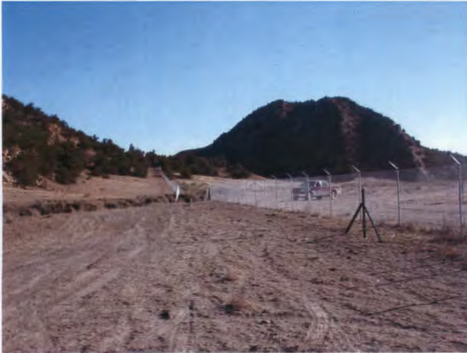
Photo 1: Chain link fence along western boundary of Parcel 3, looking north from gate location.
