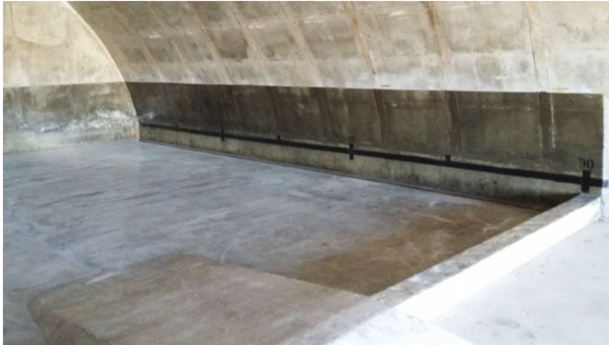
Photograph 3: Interior of Igloo B-1007 (west wall) showing secondary bermed containment and waterproof sealant. Date of Photograph: 13 February 2015
