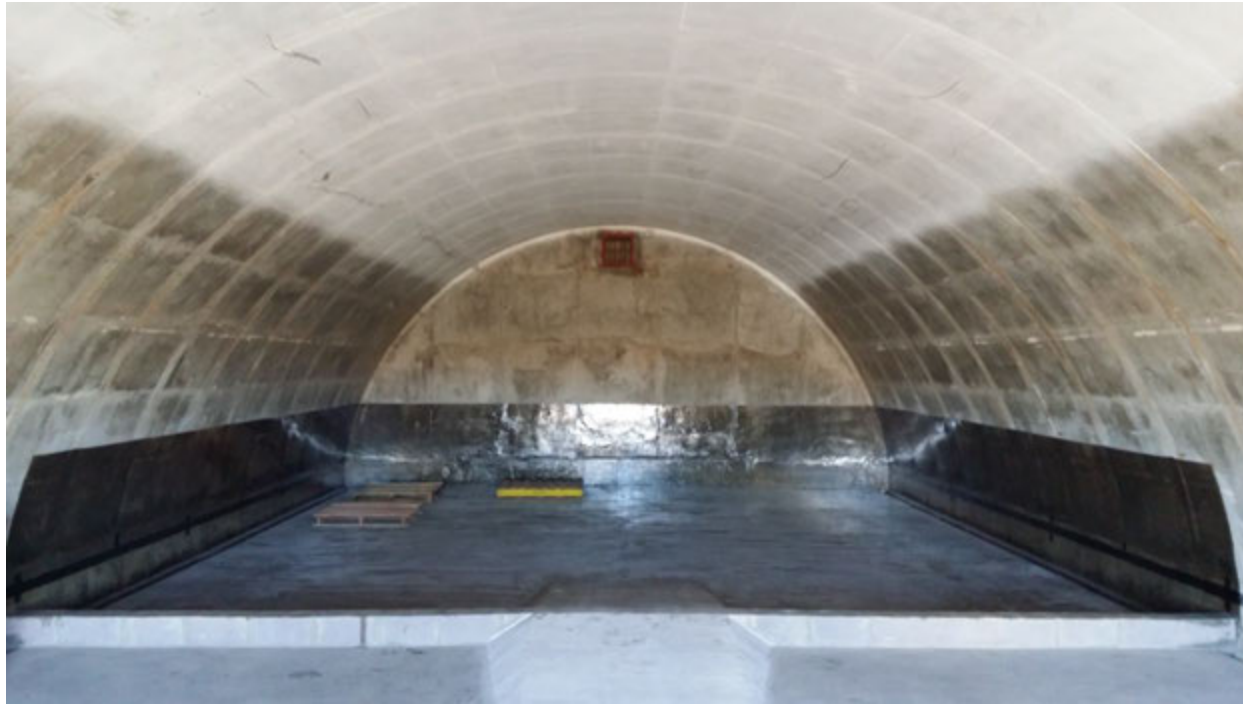
Photograph 2: Interior of Igloo B-1007 (Less-Than-90-Day holding facility) showing secondary bermed containment and waterproof sealant. Date of Photograph: 13 February 2015
