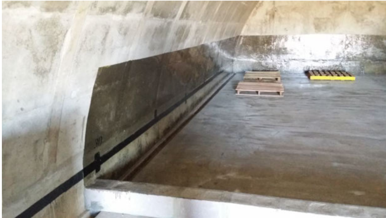
Photograph 5: Interior of Igloo B-1007 (east wall) showing secondary bermed containment and waterproof sealant. Date of Photograph: 13 February 2015
