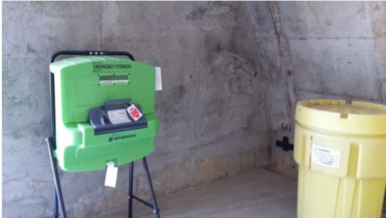
Photograph 6: Interior of Igloo B-1007, showing emergency eyewash station and drum of spill-absorbent powder. Date of Photograph: 13 February 2015
