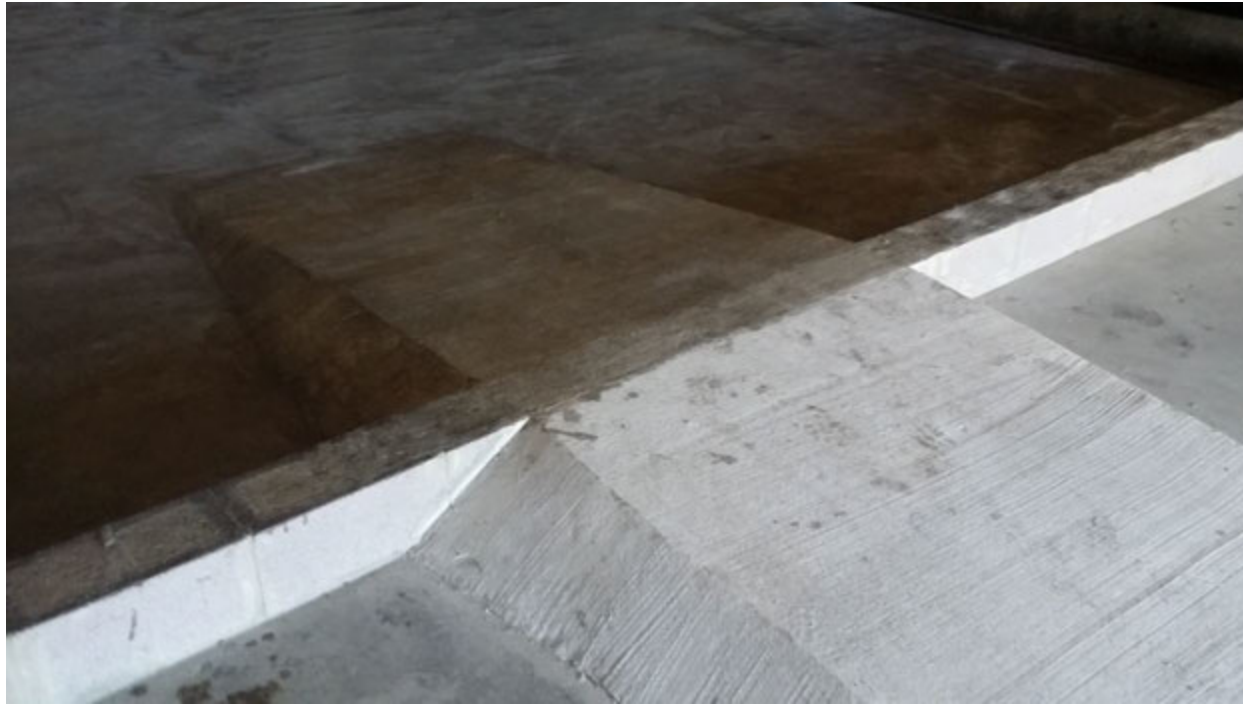
Photograph 4: Interior of Igloo B-1007 (Less-Than-90-Day holding facility) showing access ramp to secondary containment area. Date of Photograph: 13 February 2015
