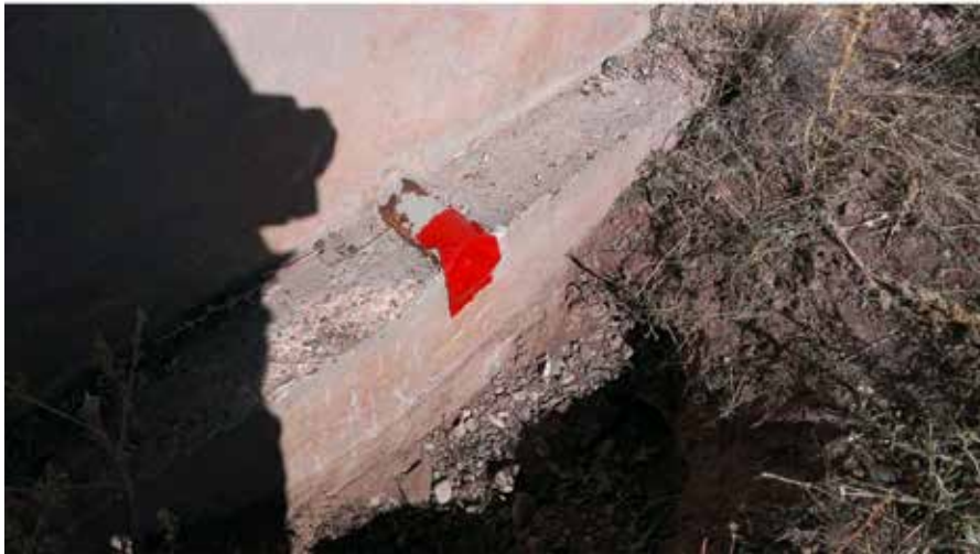
Photograph No. 14 A view of excavated soil beneath a drain pipe at Igloo C-1552.
