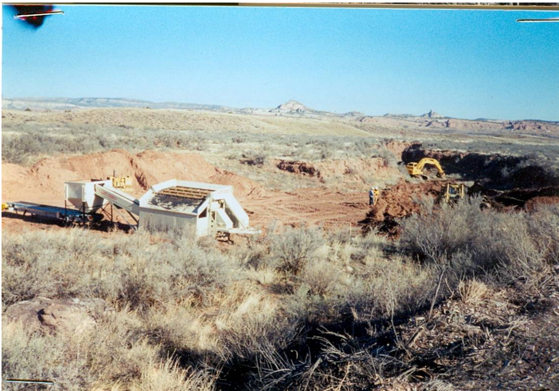
Photograph 5-2. Looking south to north of Central Landfill; screen is placed in Area D.
