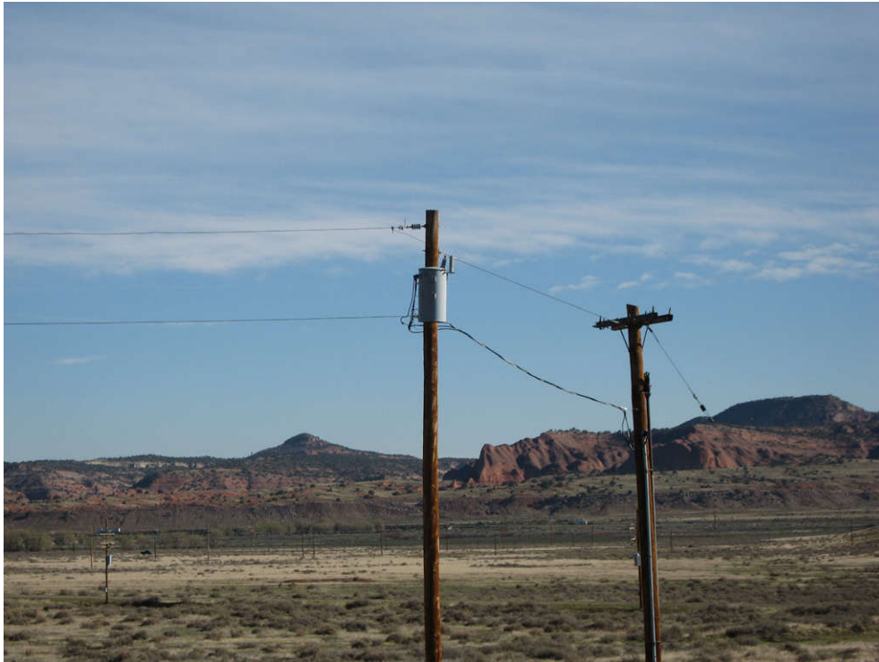
Photo 7-9: Part of AOC 75, looking north at transformer southwest of Disassembly Plant.
