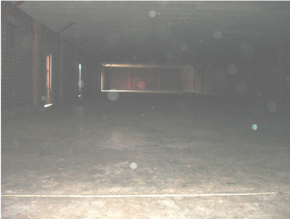
Photo 5-9: AOC 69, Standard Magazine, looking west at typical condition of interior of building.
