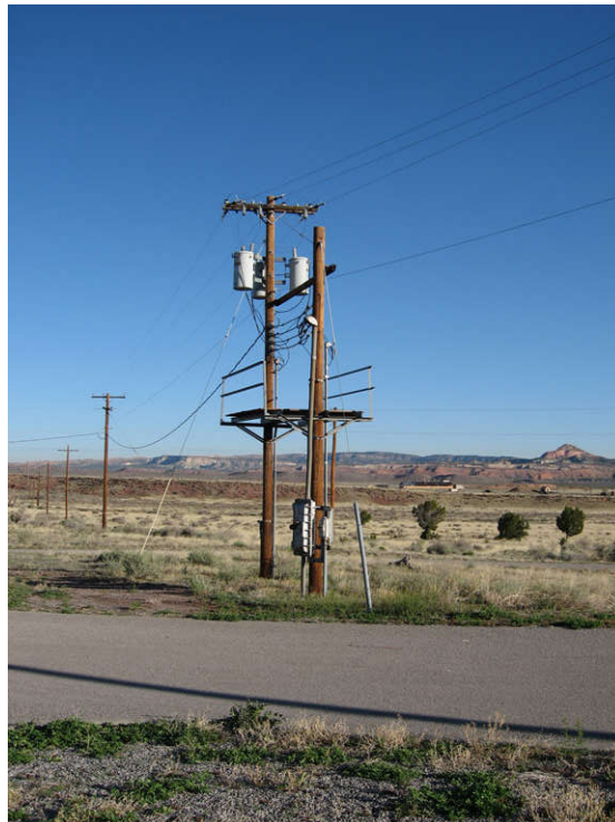
Photo 7-6: Part of OAC 75, looking northwest at second group of transformers northwest of Building 528.
