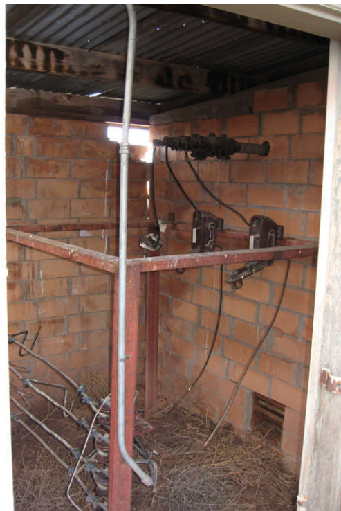
Photo 7-8: Part of AOC 75, showing former transformer pad in Building 519.
