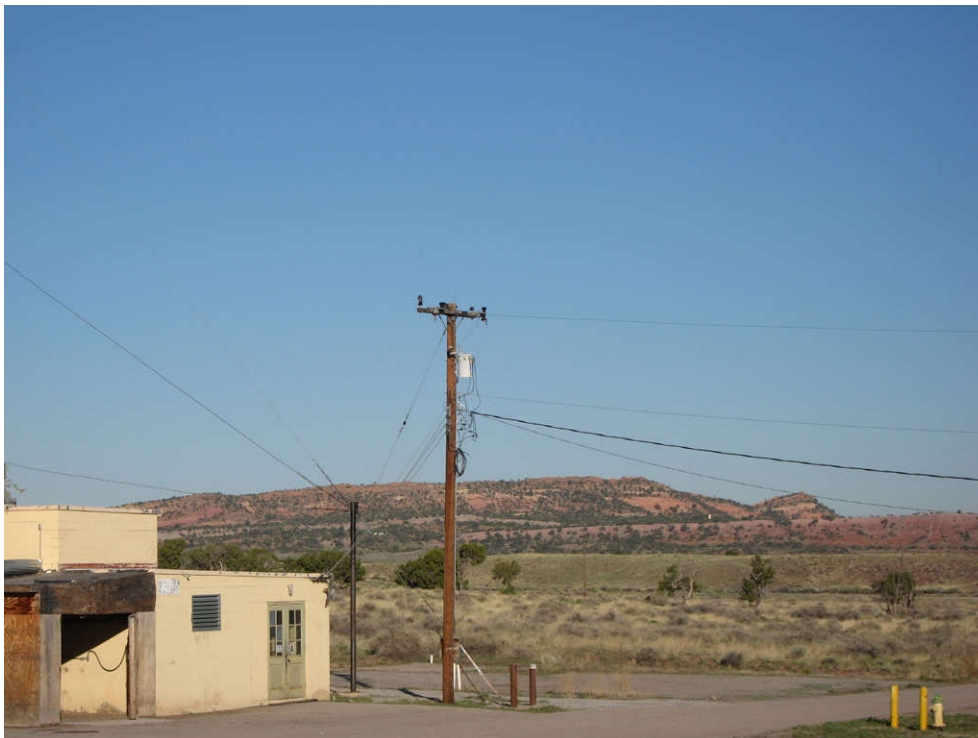
Photo 7-4: Part of AOC 75, looking southwest at transformer north of Building 527.
