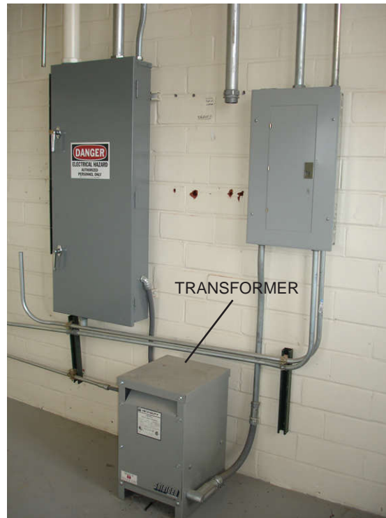
Photo 7-3: Part of AOC 75, showing air cooled transformer in Building 536.
