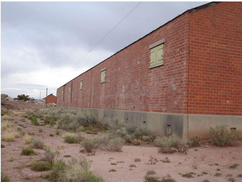
Photo 5-4: AOC 69, Standard Magazine, looking southeast at typical exterior condition of rear of building.
