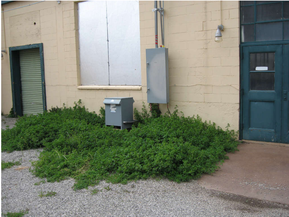
Photo 7-7: Part of AOC 75, showing transformer at south end of Building 528.
