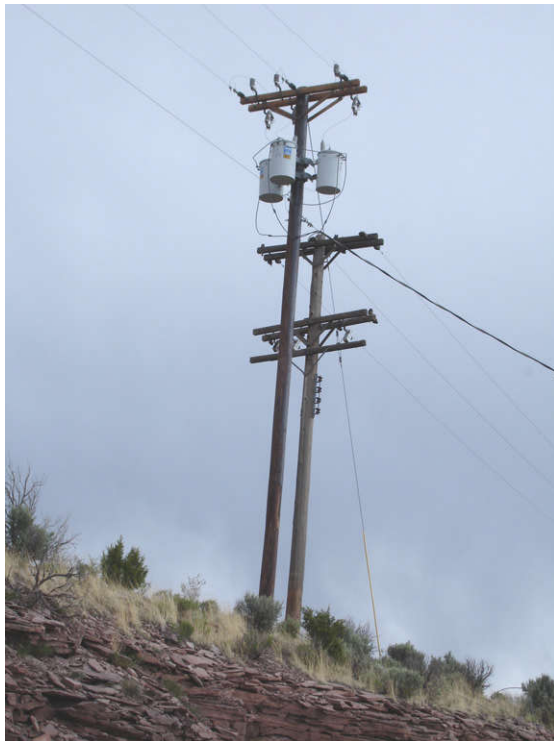
Photo 7-1: Part of AOC 75, looking southeast at transformers at Building 536.
