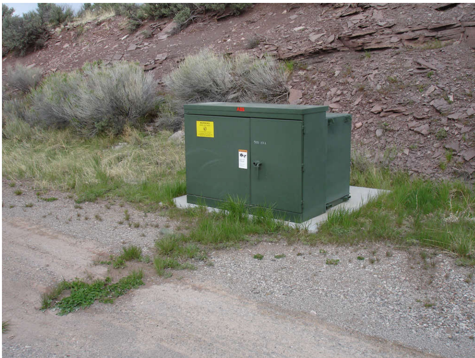
Photo 7-2: Part of AOC 75, looking northeast at transformer east of Building 536.
