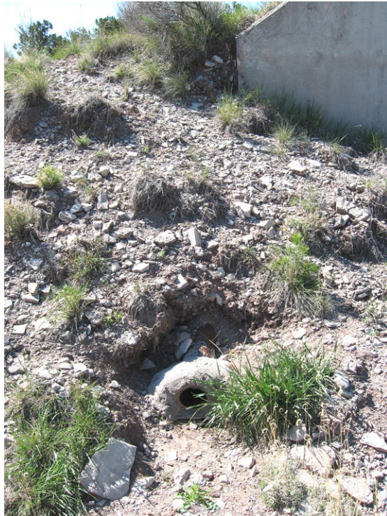
Photo 4-11: AOC 30, Igloo Block D, showing typical example of a clay drain tile (exterior perimeter drain as shown in historical drawings) observed at several igloos.
