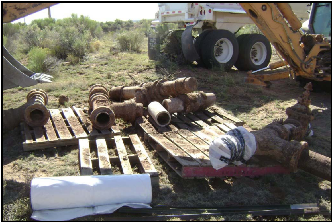
Parcel 12 / AOC 93 – Bivouac and Tank Training Area – North debris pile area removal – asbestos contaminated pipe double wrapped and sealed
