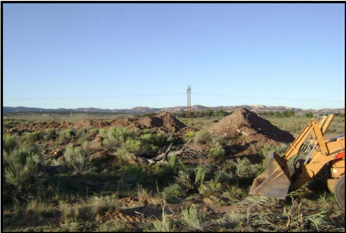
Parcel 12 / AOC 93 – Bivouac and Tank Training Area – North debris pile area removal
