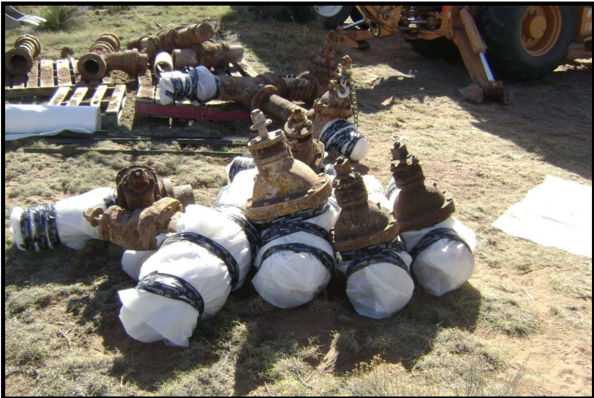
Parcel 12 / AOC 93 – Bivouac and Tank Training Area – North debris pile area removal - asbestos contaminated pipe double wrapped and sealed
