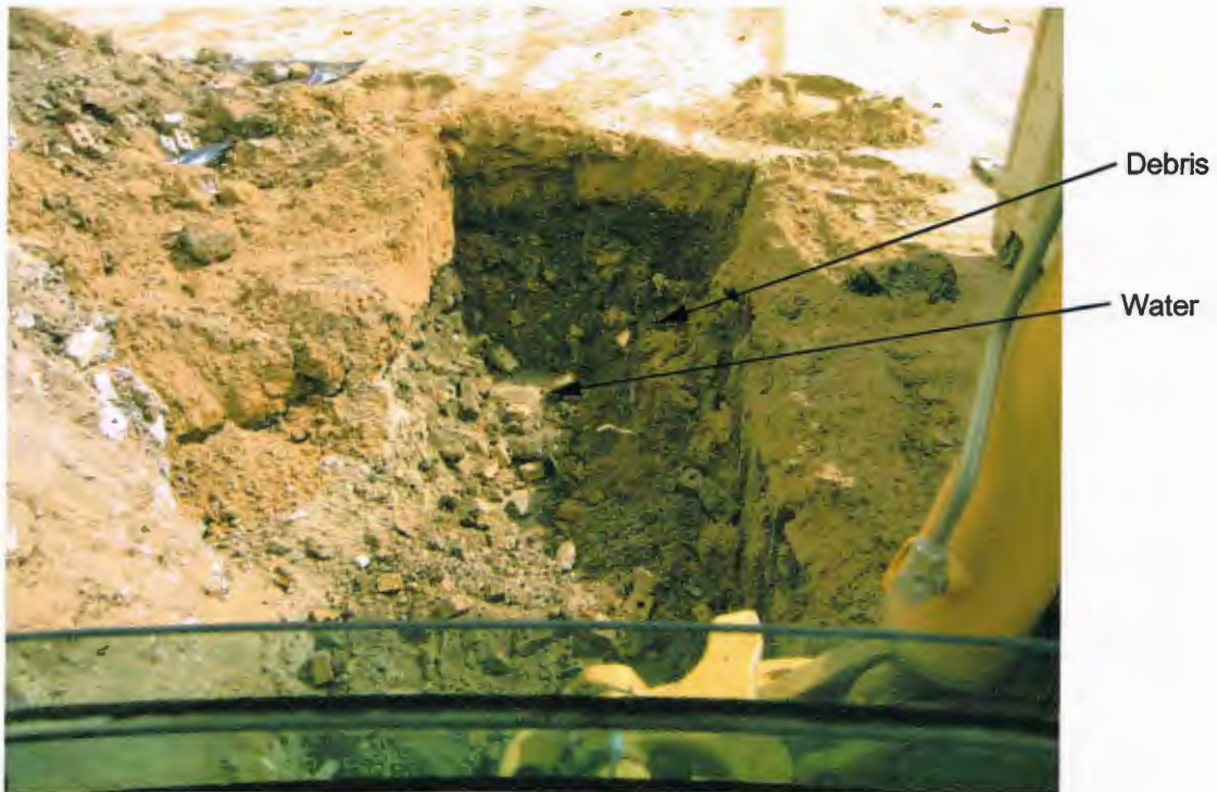
Photo 4: View to east showing water and debris.
