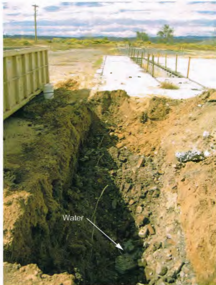
Photo 3: View to west showing excavation. Rebar in excavation is from former Building 11 footer. Note water in bottom of excavation.
