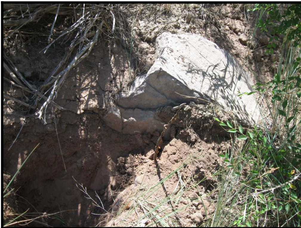
Wire Running Under Boulder Left in Grid
