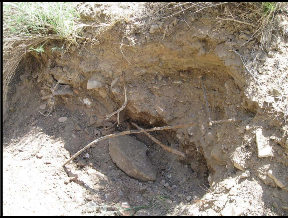
Exposed Metal Rebar Left in Place
